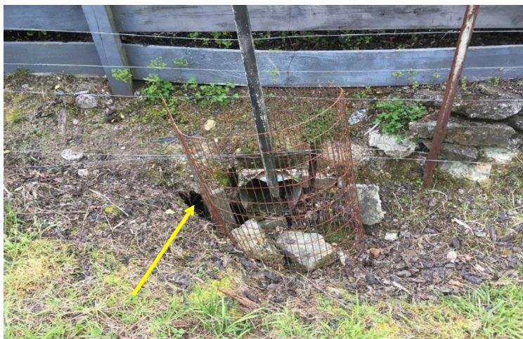
Figure 6: Photograph of pre-existing boundary-line drainage arrangements, with arrow pointing at eroded hole (taken 24 October 2019).
