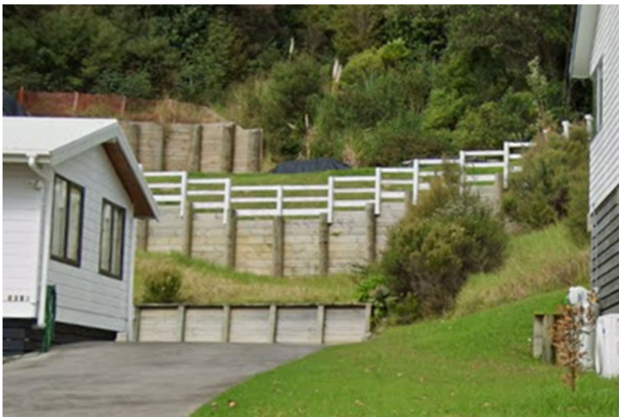
Figure 3: Photograph showing the retaining wall and barrier (taken from Google Maps on 4 August 2023).
