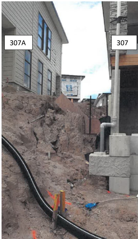
Figure 8: Scour and erosion between 307 and 307A Lakes Boulevard
