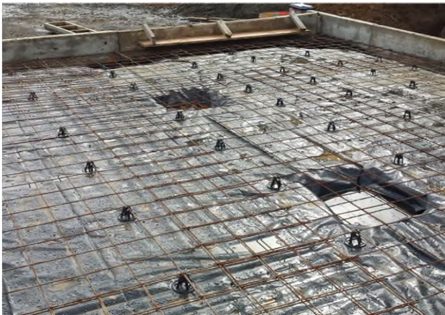
Figure 2: Photograph of excess water within the internal pads
