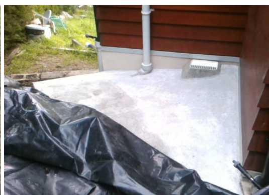
Figure 3: Sloping concrete surface to south side of ensuite extension 32
