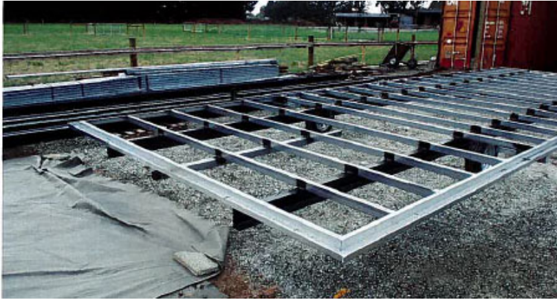
Figure 2: Photograph of a completed support frame with two wheels installed for the purpose of moving the support frame (and structure) around the yard during construction.
