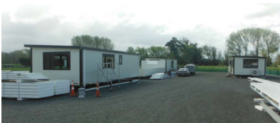
Figure 1: Photograph showing three units which are close to completion and two units in the initial stages of construction (middle left and front right). These units were observed on 02 October 2019.
