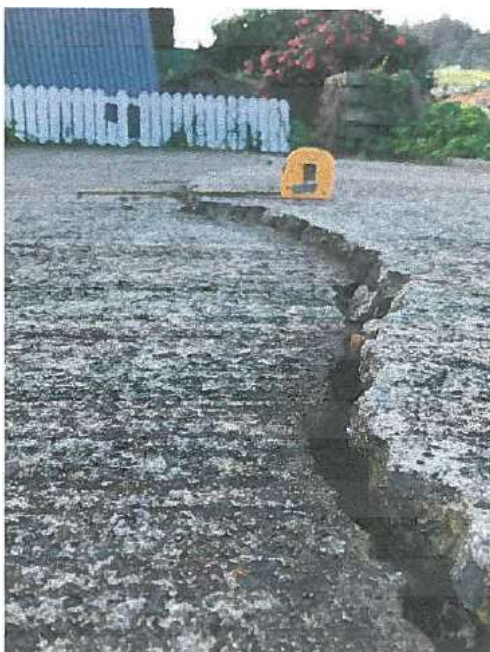
Figure 5: Photograph of driveway crack
