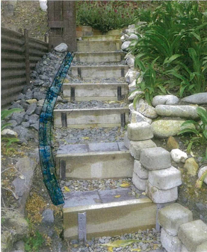
Figure 4: Image provided by the authority. Approximate location of drainage coil marked in 'blue'
