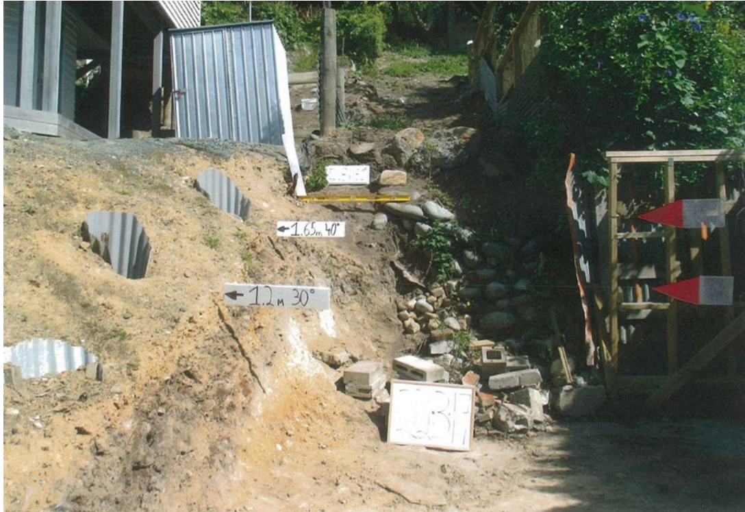
Figure 4: Earthworks on 22 March 2017 viewed from Poynters Crescent, with the applicant's property on the left (image provided by the applicant)
