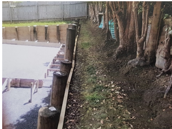
Figure 1: view of the retaining wall looking west (image taken early 2018 by the applicant's surveyor)
