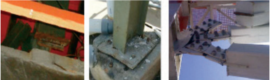
Figure 21: Weld failure of rafter attachment to concrete support (left); Base plate deformation (centre); Steel bracing cleat fracture (right)
