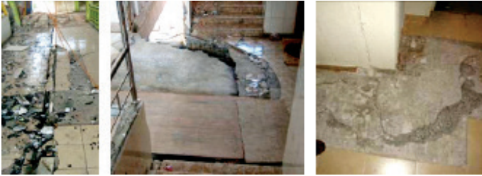
Figure 18: Structural movement joint in suspended slab (left); Floor diaphragm damage (centre); Punching shear failure in suspended slab at end of shear wall (right)
