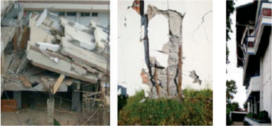
Figure 16: Weak column-strong beam frame collapse (left); Column flexural hinging with concrete crushing and reinforcing steel fracture (centre); Falling hazard from partially detached wall cladding panel (right)
