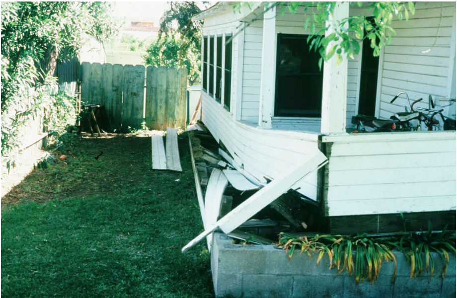
Figure 11: House fallen off its foundation (source SAP Evaluation Student Manual p34)
