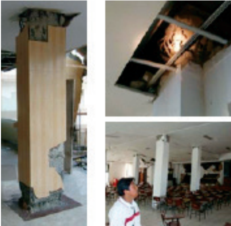
Figure 15: Column hinging top and bottom (left); Top of column hinging failure above suspended ceiling (top); Columns out-of-plumb (bottom)
