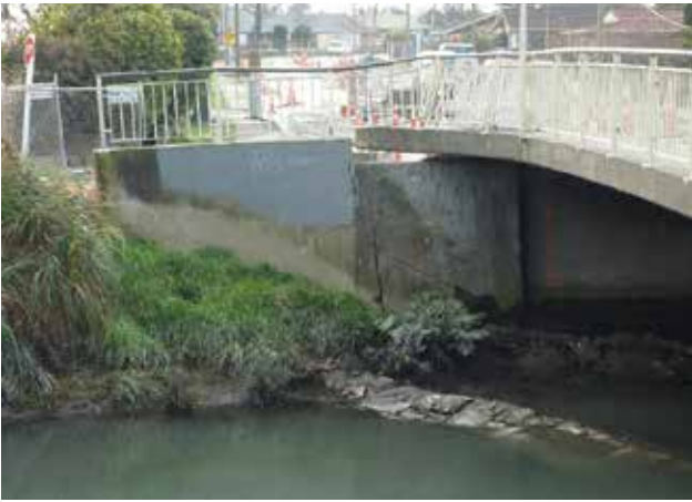
Figure 13: Lateral spreading of soil and damage to a bridge in Canterbury 2011
