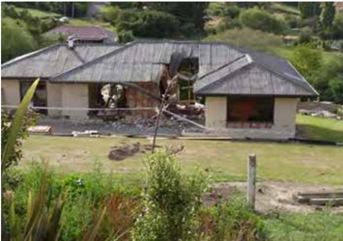
Figure 6: Boulder roll damage to a house in Rapaki, Christchurch during the 2010–2011 Canterbury earthquake sequence
