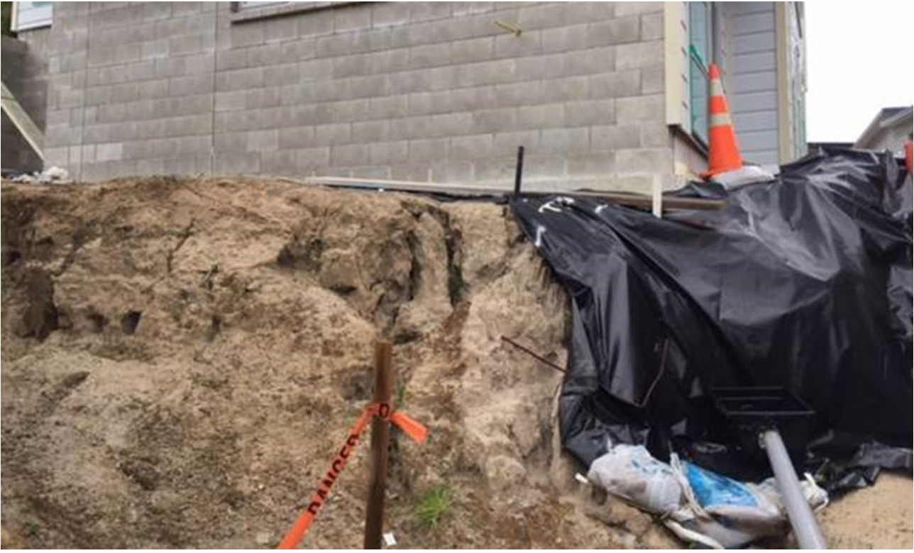
Figure 4: Unretained section of soil which provides support to a dwellings external masonry wall
