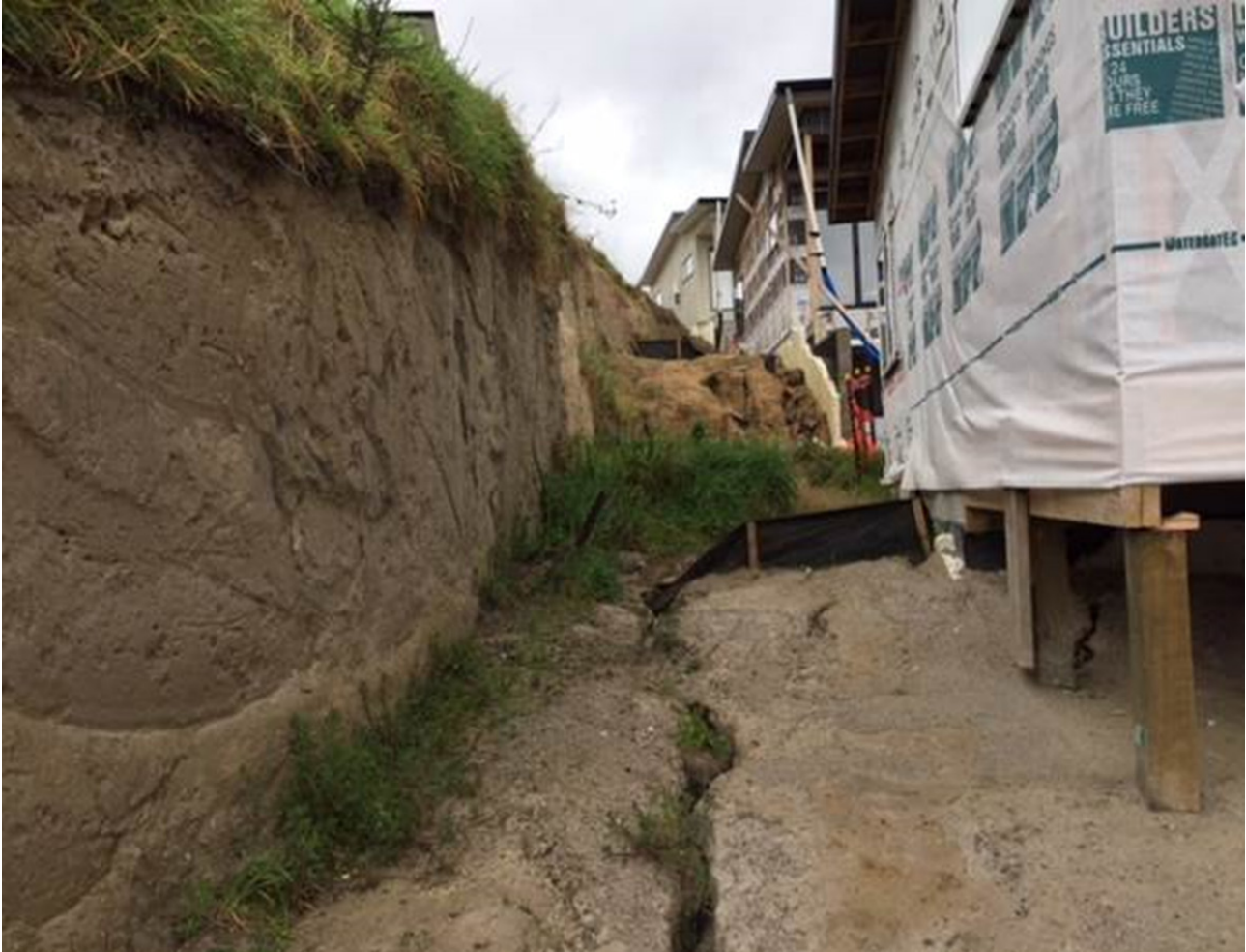
Figure 6: Example of an unretained cut along a property boundary of the Bella Vista Development.
