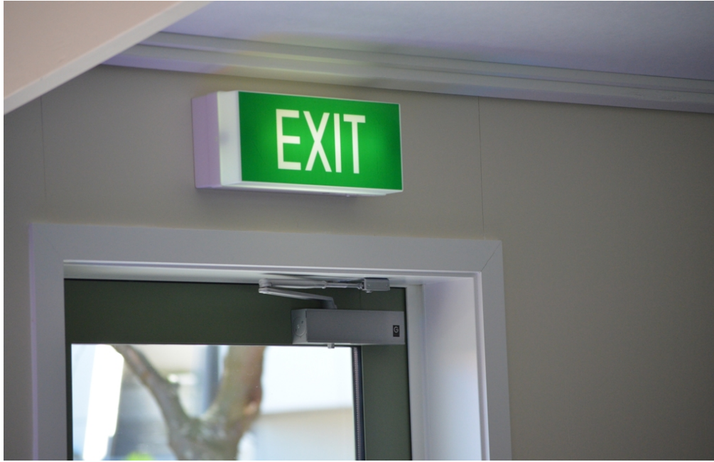
Photo 1: Emergency lighting omitted from the compliance schedule
