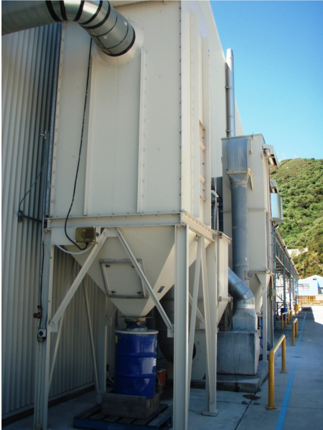
Photo 1: Dust/fume extractor to the production plant building needs to be reinstated in the compliance schedule under mechanical ventilation (SS9)
