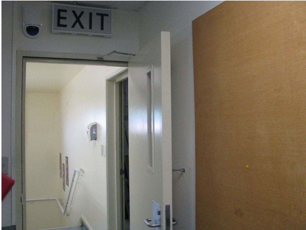
Photo 1: Mezzanine smoke-stop doors held open by cabin hooks
