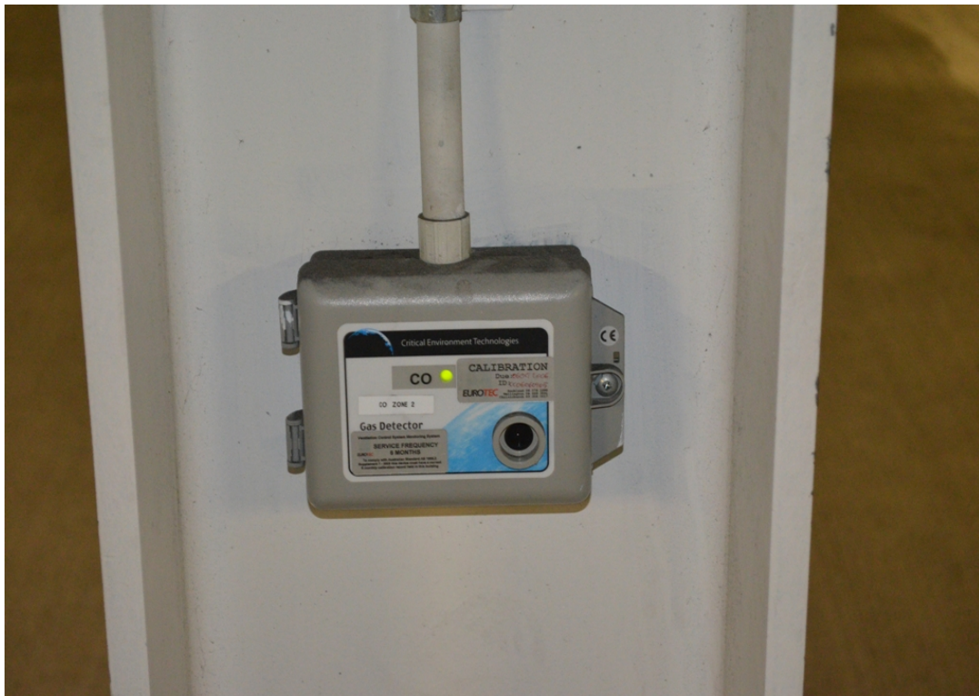
Photo 1: Carbon monoxide detector system omitted from compliance schedule
