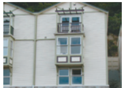
Three storey (SR) residential dwelling with an E2/AS1 risk score of 15 (vertical plane fire separation only)
