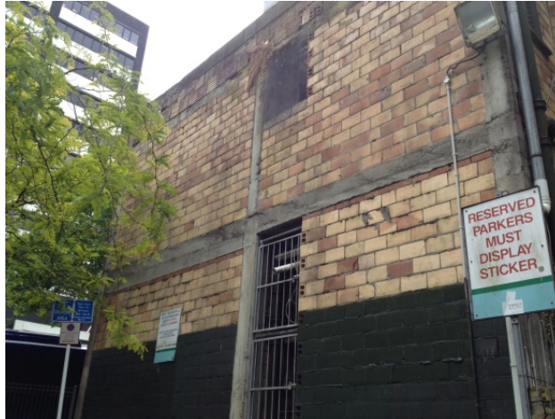
Figure C7.3: Example of a reinforced concrete frame with terracotta masonry infill (Kevin Walsh)
