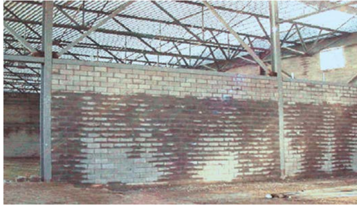
Figure C7.5: Examples of steel frame industrial building with concrete block infill (David Biggs)
