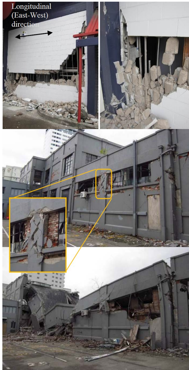
Figure C7.8: Masonry infill frame damage observed following the 2010–2011 Canterbury earthquakes (Kam et al., 2011)
