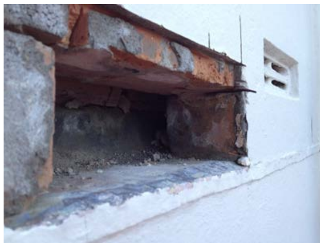
Figure C7.2: Typical clay brick cavity infill wall construction with plaster façade and single brick removed, exposing the air cavity separating two single wythes of clay brick (Kevin Walsh)
