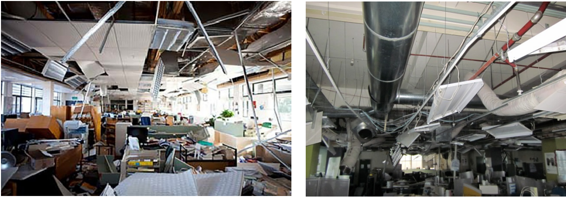
Figure C10.2: Ceiling and other damage (Dhakal, 2010 and McGuigan)
