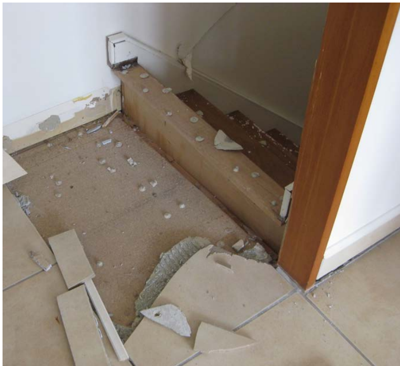
Figure C10.6: Stair that has sheared connections to the floor on a timber framed structure and ridden up above the floor (BRANZ)
