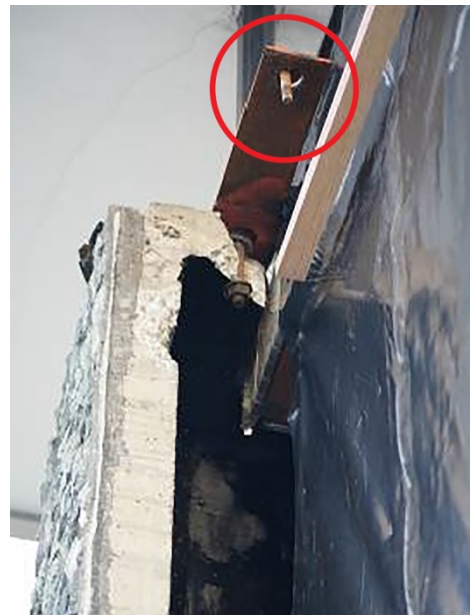
Figure C10.1: Failure of a precast concrete panel (Baird et al., 2011)
