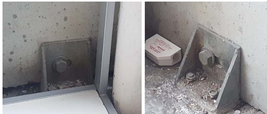
Figure C10.3: Precast connections with no remaining sliding movement allowance to accommodate inter-storey drift (Baird et al., 2011)
