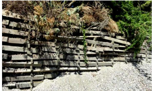
Figure A.4: Damaged timber crib wall
