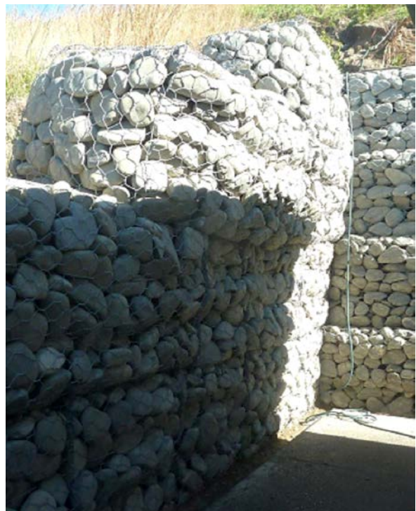
Figure A.6: Gabion wall showing bulging and outwards movement
