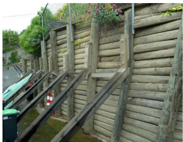
Figure A.3: Damaged timber pole wall showing failure of poles at anchor location and failure of anchors
