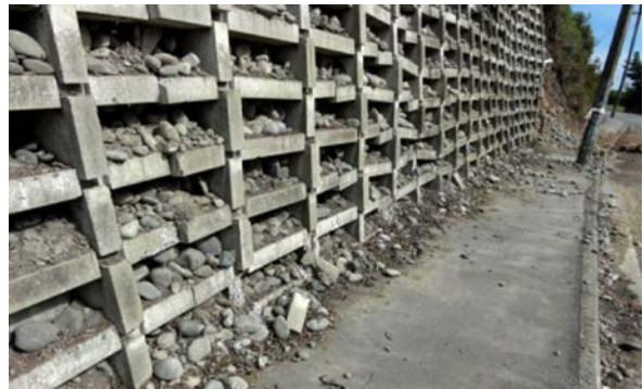
Figure A.5: Concrete crib wall showing loss of rounded gravel backfill
