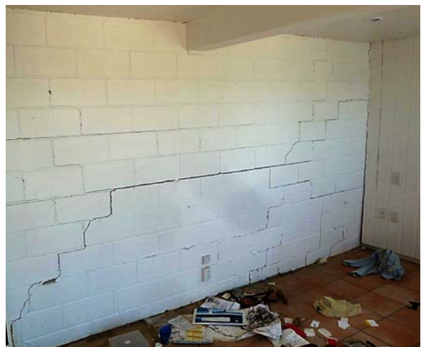
Figure A.2: Damaged concrete block basement wall
