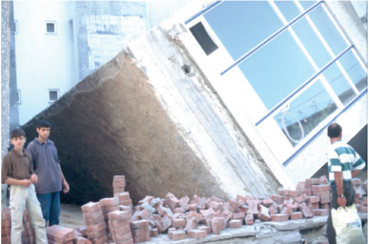
Figure 5.5: Instability of a tall building on a raft foundation during the 1999 Kocaeli earthquake
